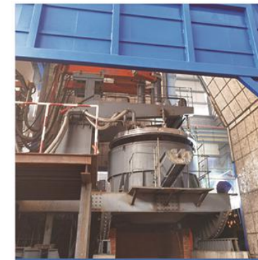
25吨电弧炉 25 tons Electric-arc furnace
